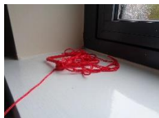
The alarm cord is not accessible.
